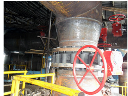
McCannalok Series 41R installed in sugar mill operation.
