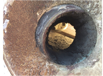
After 2 months in service, a competitor's valve showed signs of upstream severe media buildup — causing frequent leaks and lockups.
