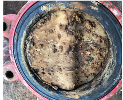
This butterfly valve, used for isolation, shows an example of the encrusted, abrasive media.
