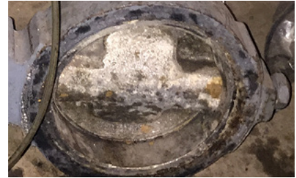
The existing butterfly valves showed signs of heavy sugar crystal deposits, making the valves inoperable after as few as 15 days of service.
