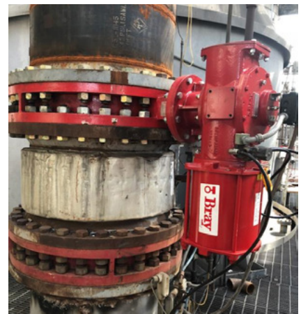
Bray automation solutions performed continuously for more than 700,000 cycles in the harsh sugar processing environment.
