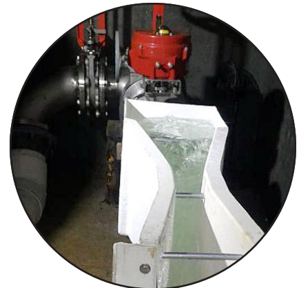
Parshall flume metering device used to measure flow of surface water.
