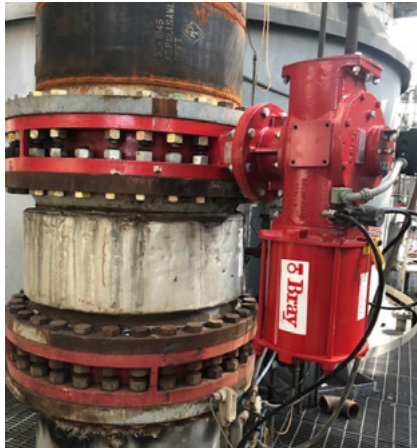
Bray automation solutions performed continuously for more than 350,000 cycles in the harsh environment.
