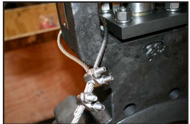
Figure 4: Wire rope secured around the neck of the valve.
